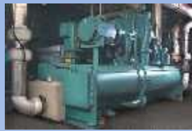
Compressor for cooling
