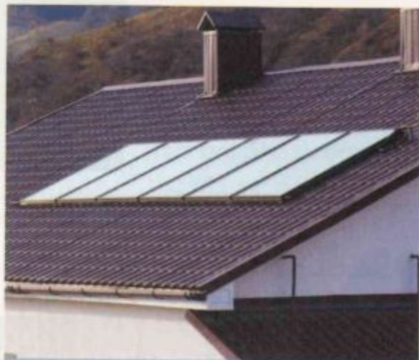
Photovoltaic solar panels
