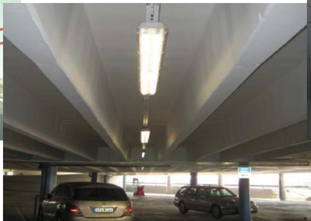
Low bay lighting
