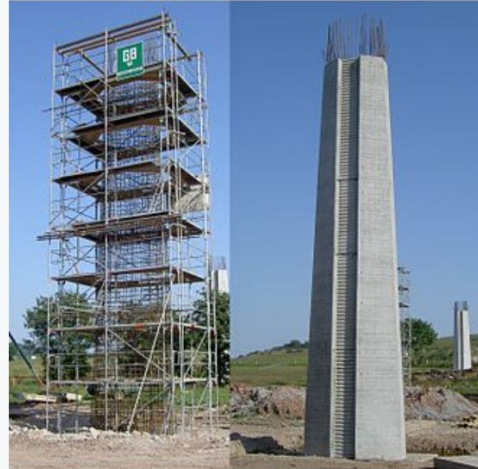
A heavy, reinforced concrete column, seen before and after the concrete has been cast in place around its rebar frame
